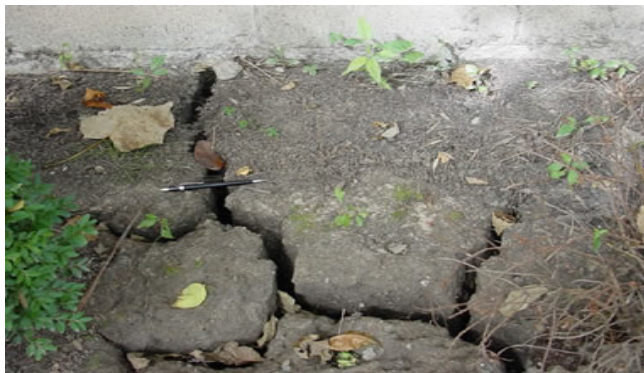
Figure 1: Cracks in Expansive Soil.
